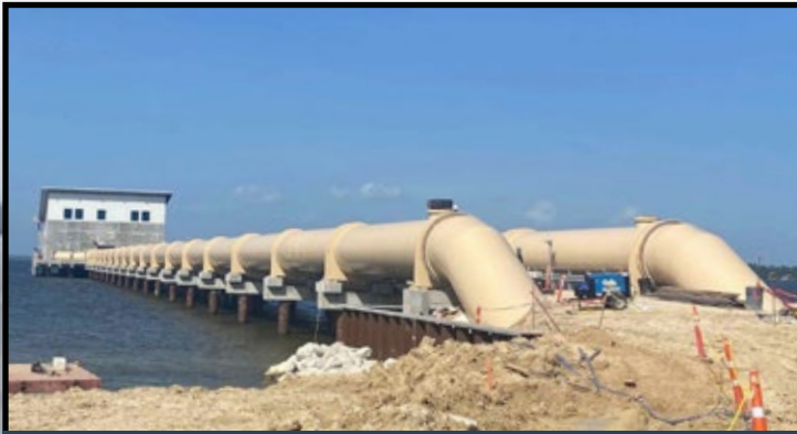
The pump station is connected by a bridge with dual 108" Raw Water Pipelines running on each side of the bridge.
